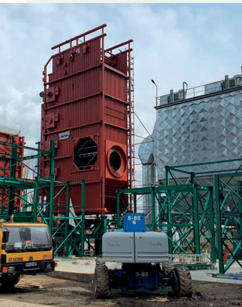
Cogeneration plant Expur, Romania
